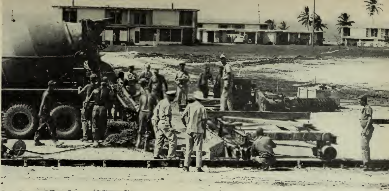
HOME WORK —Peacetime jobs of Navy Construction Battalions included housing projects such as this on Guam.
